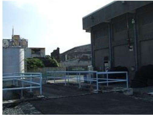
Pumping station constructed by this project
