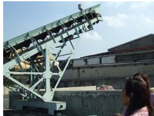
Waste processing machine in a pumping station constructed by the project
