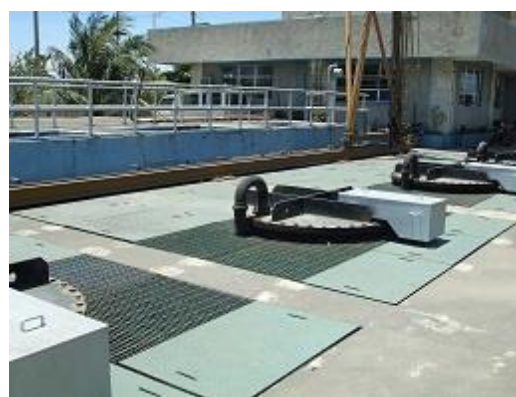
Pumps in a MMDA's pumping station, West Manggahan
