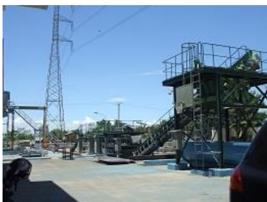
MMDA's pumping station West Manggahan
