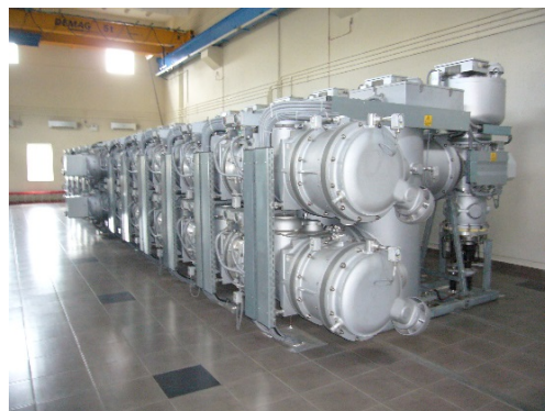
Kelanitissa Substation (inside)
