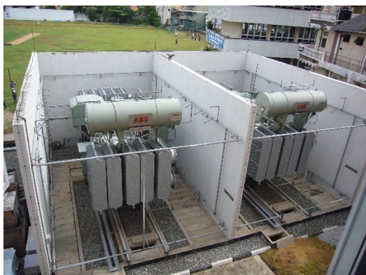
Primary Substation “H” (Outside)
