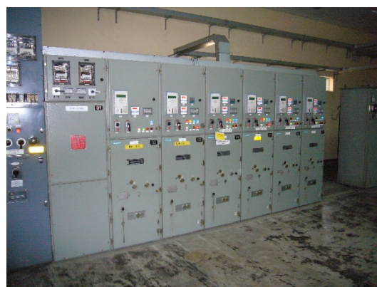
Primary Substation “H” (Inside)
