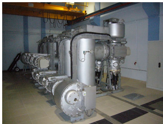
Inside of Substation “C”
