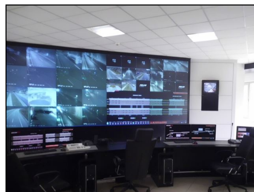
Photo 5: Control Centre of Tunnel
