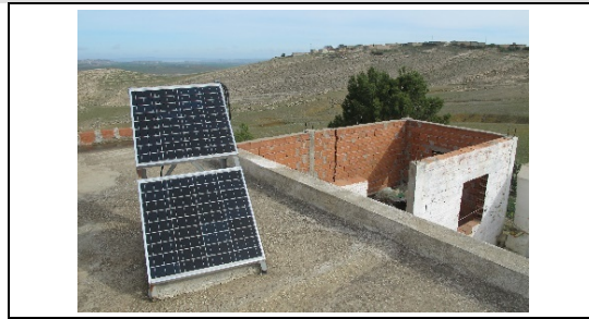
Solar panels installed in the project (Siliana Governorate)
