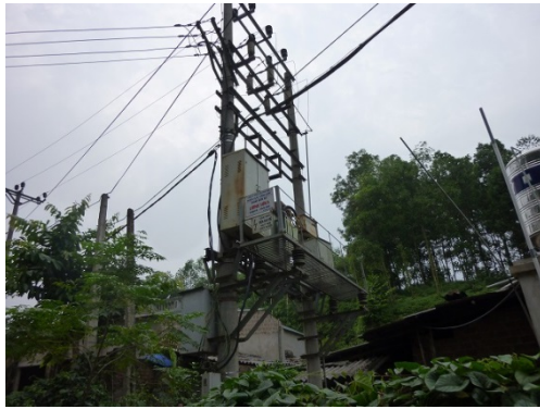
Photo 3: Installed Electricity Distribution Facility (Yen Lap District in the Phu Tho Province)
