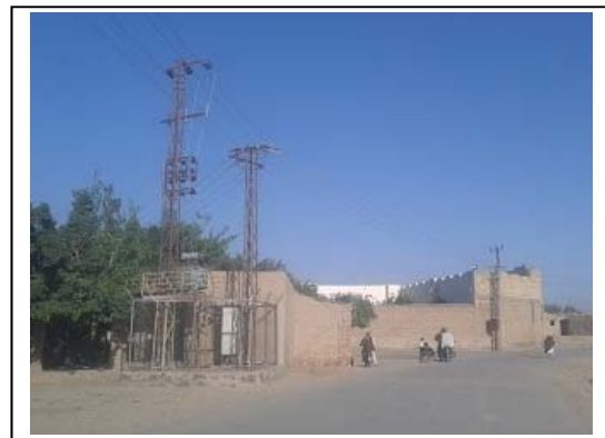
Extension of Power Supply Lines (Karz CCDC, Kandahar)
