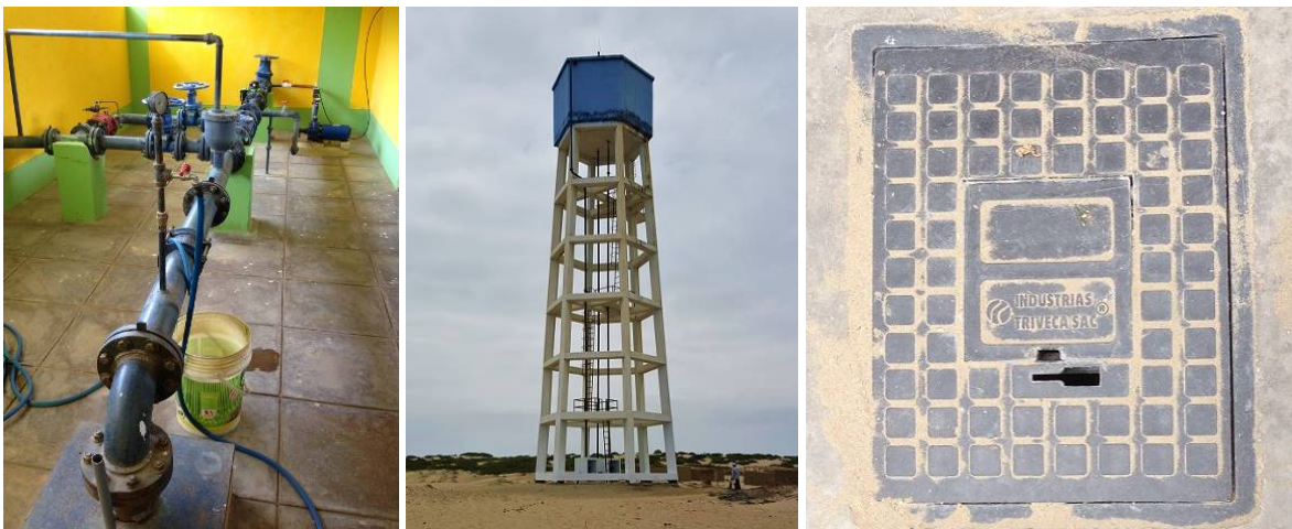
Rural water supply facility constructed by pilot projects (from left): well (Lynas, Piura Region) water reservoir (San Pablo, Piura Region) water meter box (San Pablo, Piura Region)
