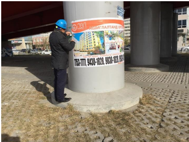
Daily inspection and cleaning Removing a business poster (At the time of ex-post evaluation)
