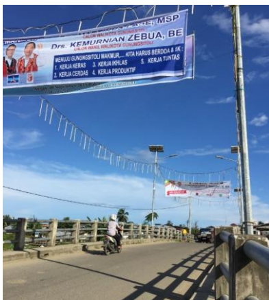
Nou A Bridge in Gunung Sitoli City (at the time of the ex-post evaluation)
