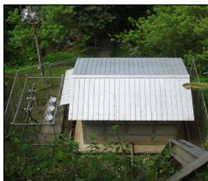
Power Generation Facility (Seasir)
