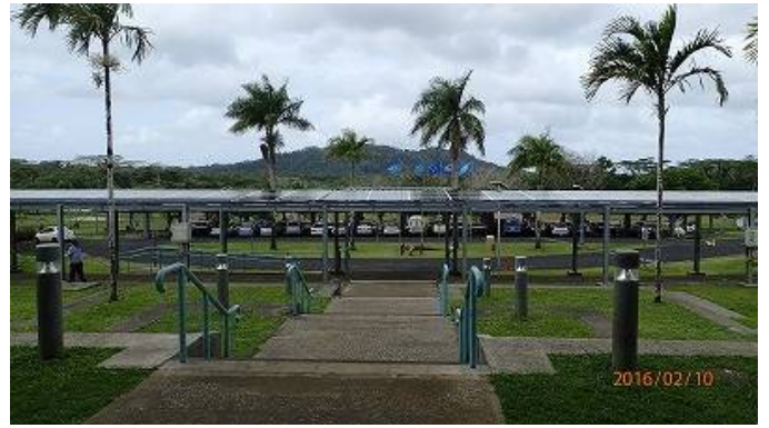
The PV system on car parking roof of COM-FSM (Palikir campus)
