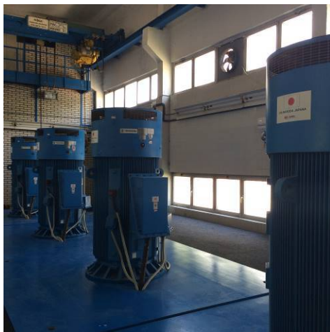
Four pumps at Mareza 2 pump station
