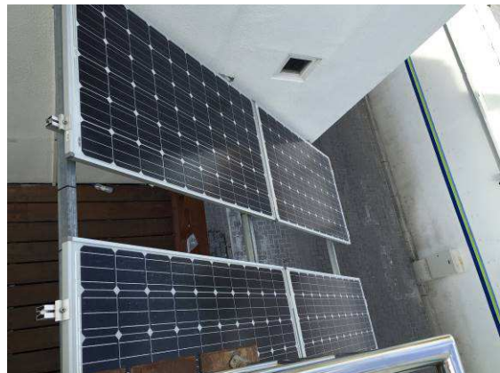
MEE's Self-Financed Solar Panels (Building of MEE)
