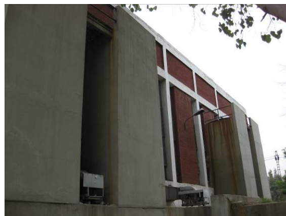
Drainage Basins (Multan Road Pumping Station)
