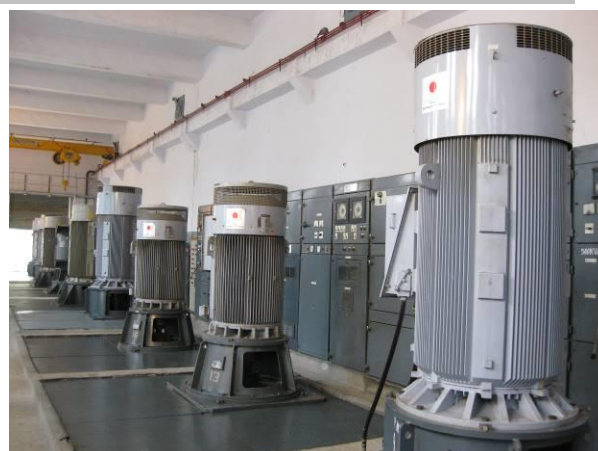
Operation and Electric Room (Gulshan-E-Ravi Pumping Station)
