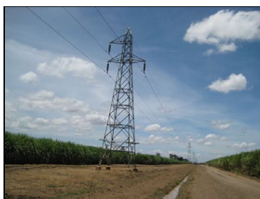
66kV Transmission Line
