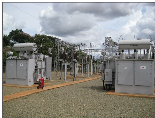
Makuyuni Substation newly installed by the project
