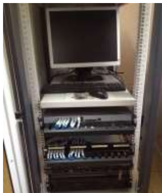
CBT installed at DCA's training center
