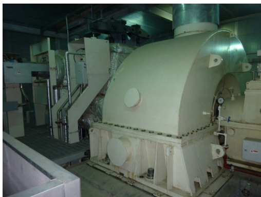
Photo 3: Gas Turbine Generation Facility
