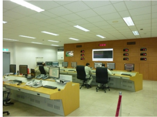
Photo 2: Central Control Room
