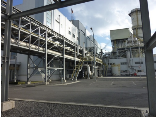
Photo 1: Inside the Yerevan CCPP
