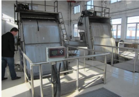
Inlet filter of the Zhanggaiying
