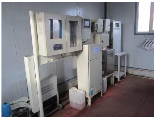
Water quality monitoring equipment at the Songpu sewage treatment plant
