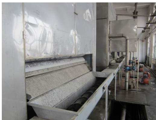
Sludge treatment facilities at the Pingfang sewage treatment plant
