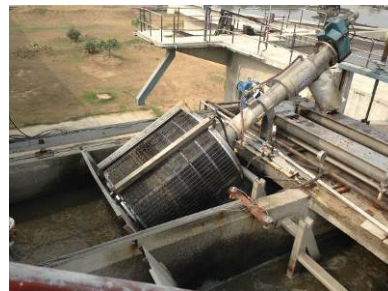
Sewerage Treatment Plant (Keshopur)
