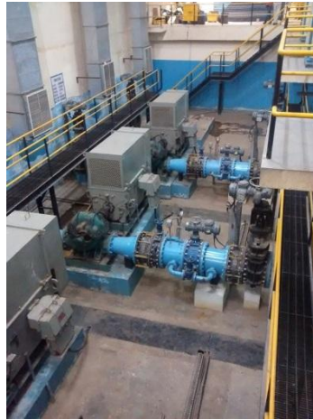
Mansarovar pumping station
