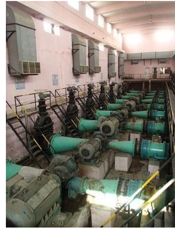
Ramniwas Bagh pumping station
