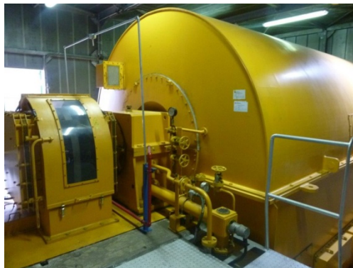
Turbine in the Power Plant
