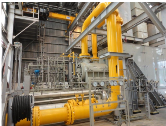
Gas Compressor (Pagardewa)
