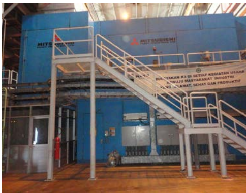
Facility where Gas Turbine is Installed
