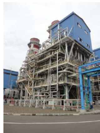
Heat Recovery Steam Generator
