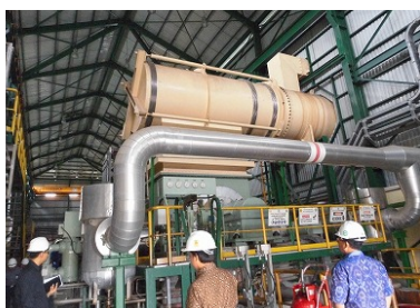
Geothermal Turbine (above) and Generator (below)
