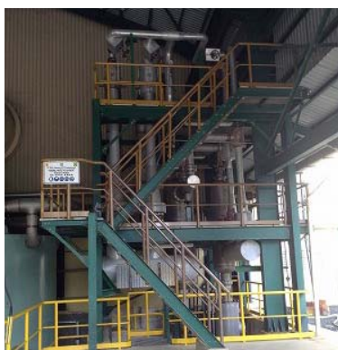
Gas extractor for Lahendong Unit 3
