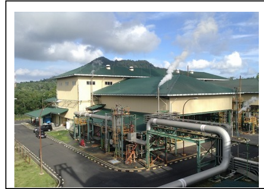
Lahendong Geothermal Power Plant
