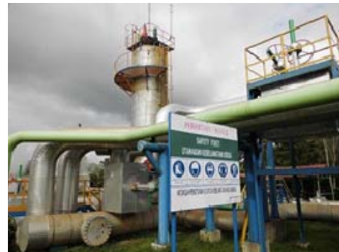
Exchange point of steam pipeline (No.23/No.28)
