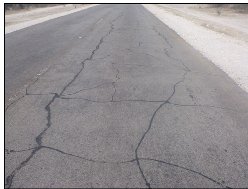
Surface cracks (after repair works, near Bunya)
