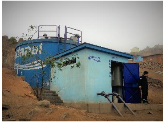
Distribution Reservoir constructed by the Project
