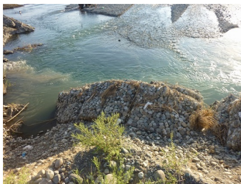
Photo 3: Gabion Fell Down due to Typhoon Koppu of 2015 (Region I: Ilocos Norte)
