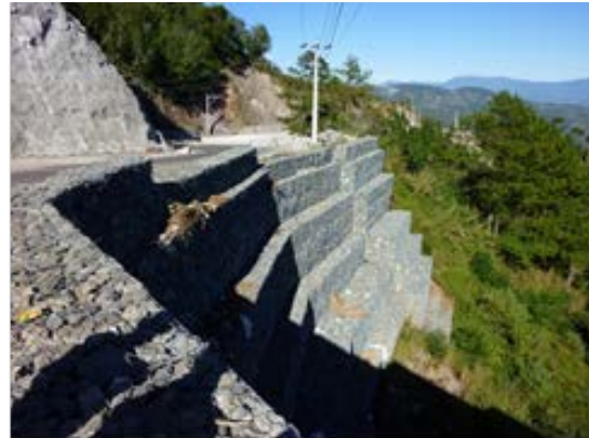
Gabion Developed Along the Road in the Mountainous Region (Benguet)
