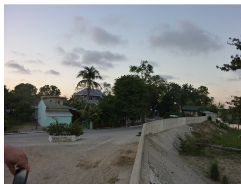
Photo 4: Functional Revetment Wall along the Residential Areas (Region I: Ilocos Norte)
