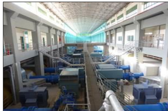
Melen Pumping Station
