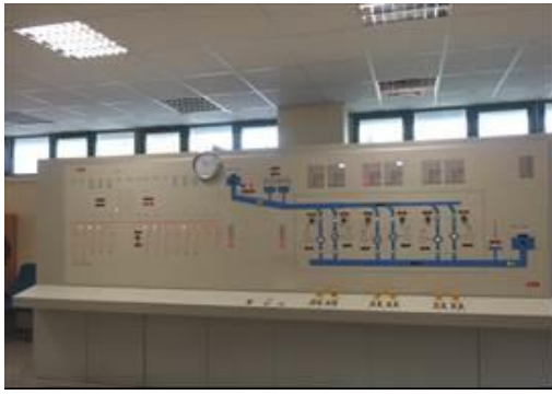
Control Room in the Treatment Plant
