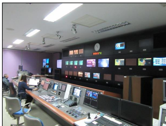
Control Room Developed in This Project
