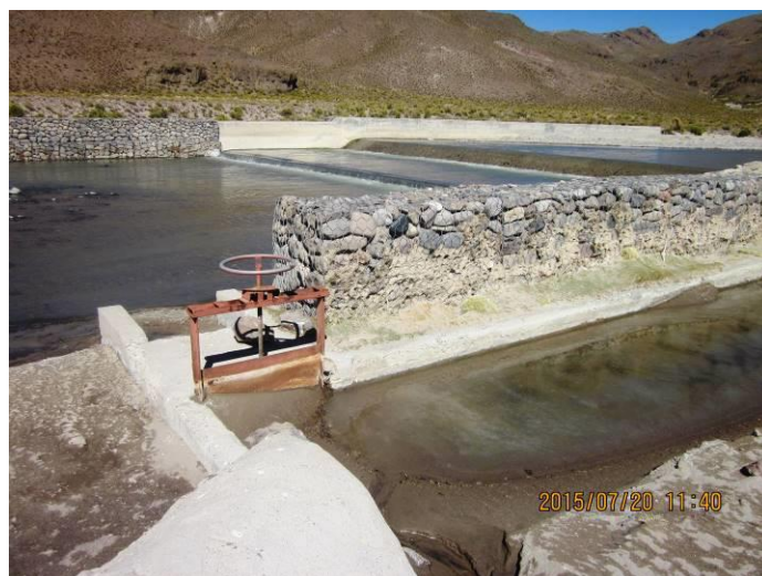
(Irrigation Facility in Turco – community of Macaya)
