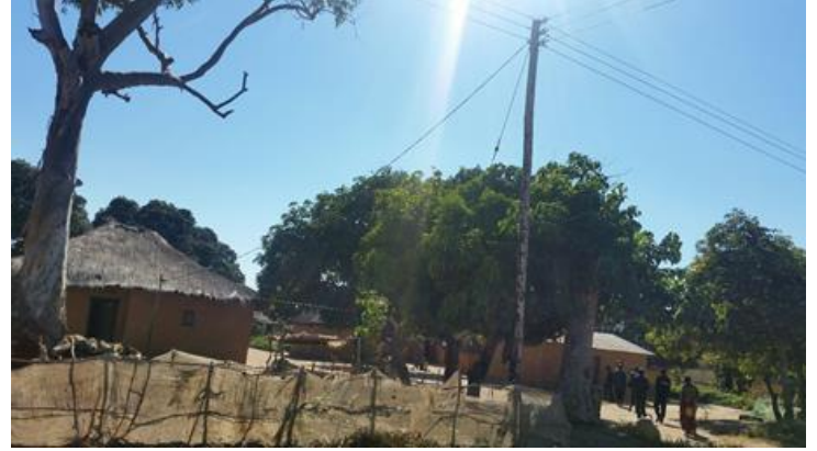
Solar PV system installed in rural Samfya.
