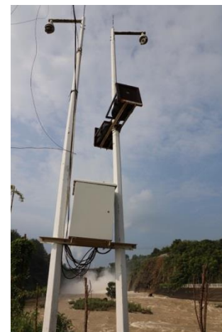
Warning system at Lushui Dam
