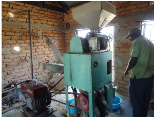
Rice milling machine installed in the building
