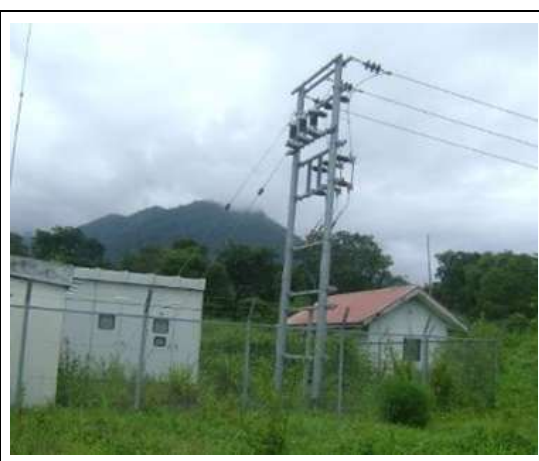
Booster Station and Distribution Line
