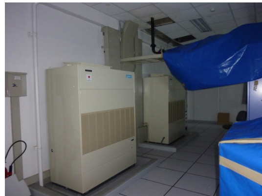
Photo 2: Water leakage sometimes occur from cracks in the ceiling caused by typhoon Nock-Ten
