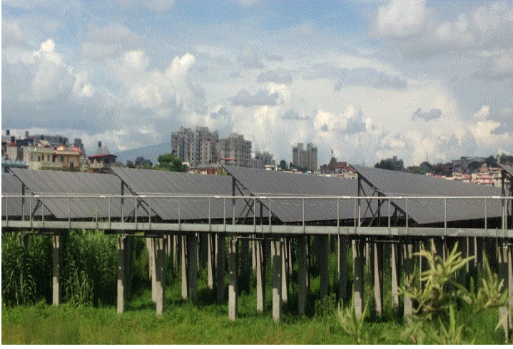
PV panels at site
