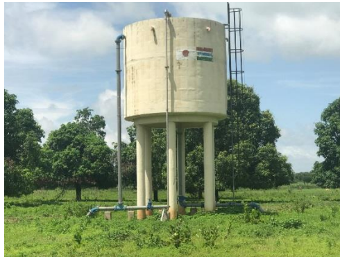
Water tank of the water facility
