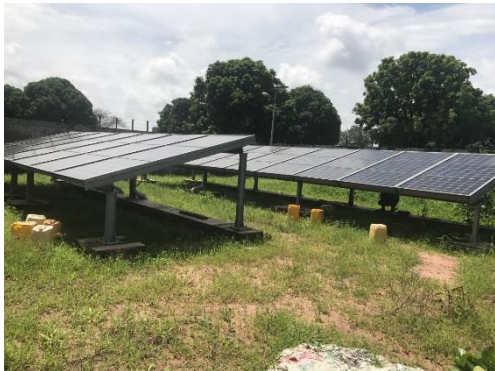
Solar panel of the water facility
