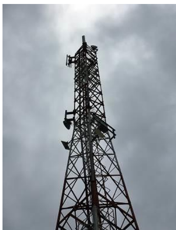
Meteorological Data Communication System (Vaisala)
