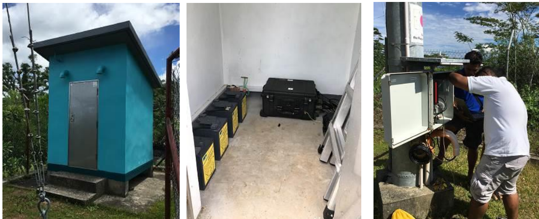
(Left) Concrete shelter: repainted wall by SMD (Togitogiga observation point) (Centre) Inside the concrete shelter: Batteries (Left), Indoor units (Centre), IP phone (Mt. Talu observation point) (Right) (Right) SMD staff working to maintain the data collection system (Le Piu Tai observation point)
