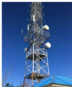
(Photo: right) Antenna Tower of the FM Transmitting Station at Simbhanjyan
