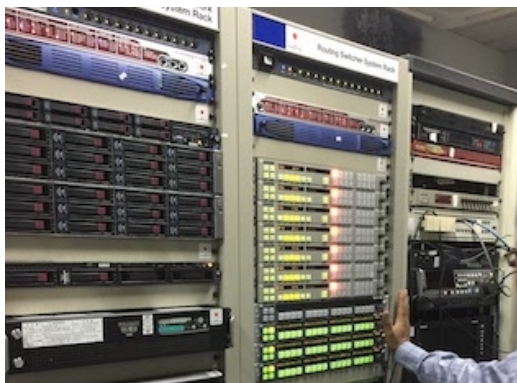
Video server (left) and routing switcher (right)
