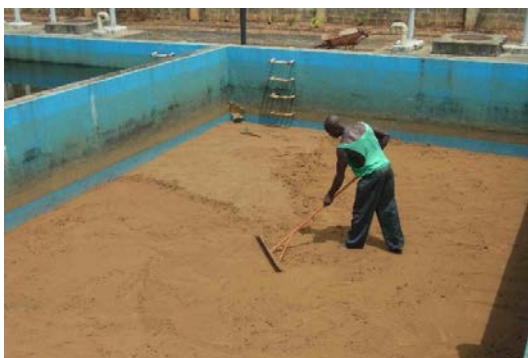
Maintaining sand in a slow sand filter basin
