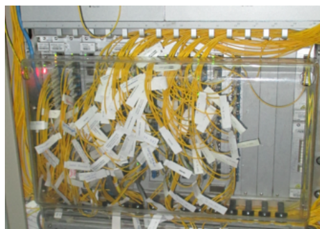
At the ex-post evaluation: Destinations of the cables can be identified easily as there are labels and the cables are bundled as needed. (The photo was taken by the external evaluator)
