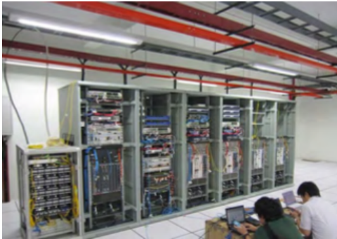
Equipment for improving internet access in Mandalay
