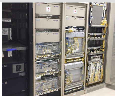
Equipment installed by the project (Nay Pyi Taw)
