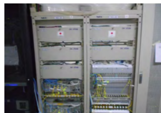
Redundant switching system for metro ring network (Yangon)
