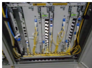
Redundant switching system for backbone ring network (Nay Pyi Taw)
