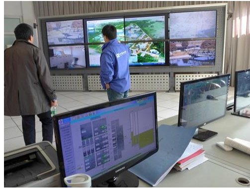
Control Room in the 7 th STP
