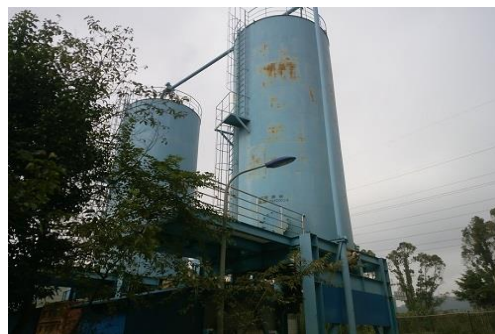
Deodorization Facility (the 4 th STP)
