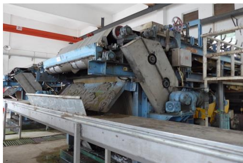
Sludge Treatment Facility (the 1 st STP)
