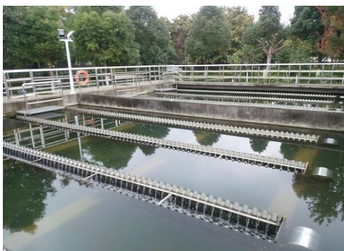
Reaction Tank in the 5 th STP
