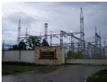
Figure 2 the Stun Hav 230/22kV Transmission Grid Substation
