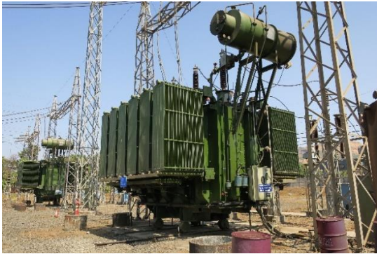
Transformer (Lonawala Substation, Pune Zone)
