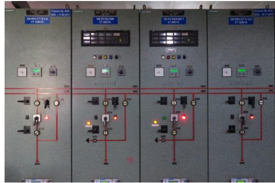
Control Panel (Kalwa Substation, Vashi Zone)
