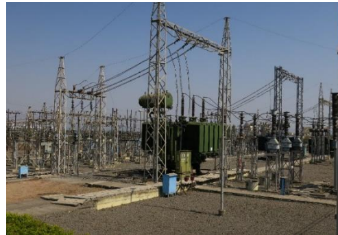
Substation Equipment Augmented by the Project (Shirwal Substation, Karad Zone)
