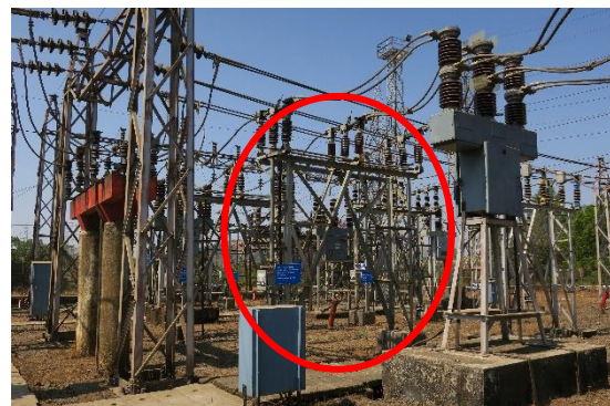
Isolator (Lonawala Substation, Pune Zone)
