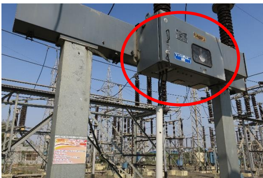
Circuit Breaker (Takali Substation, Nasik Zone)
