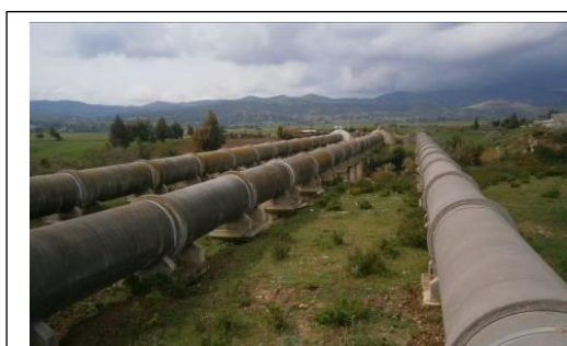
Triplicated Water-supply Pipes (along the Medjerda River)
