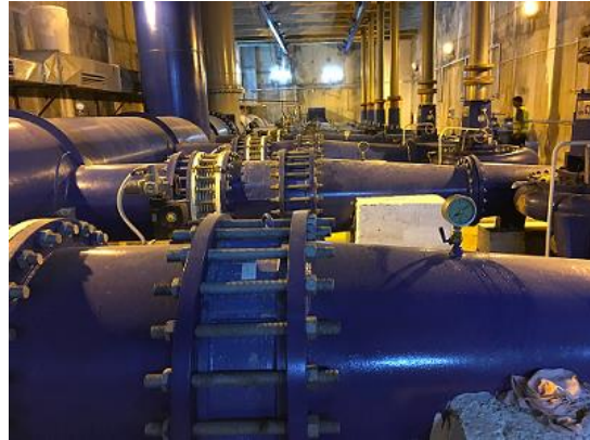
Joumine Pump Facility
