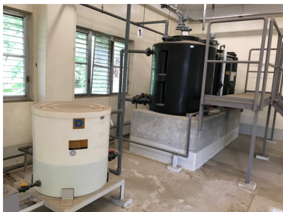
Unused chlorine facility (Tasahe Pump Station)
