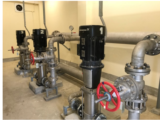
Water Transmission Pump Installed through the Project
