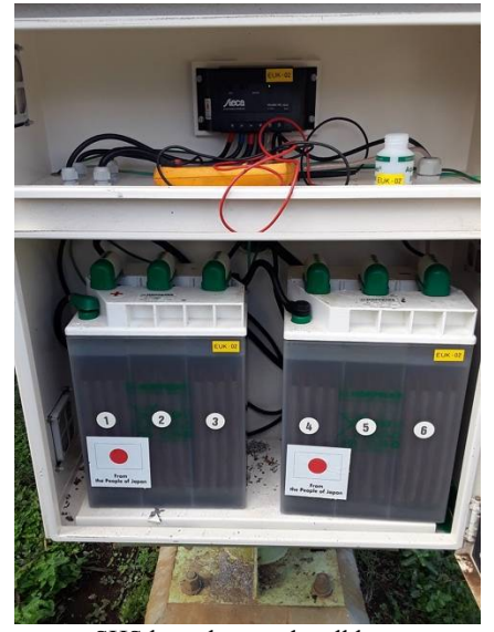
SHS box clean and well kept
