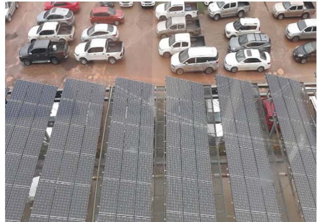
(Top view of PV system)
